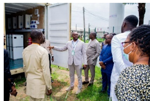
ECEWS CEO Dr. Andy Eyo inspecting the solar system at the PCR Lab in UUTH
